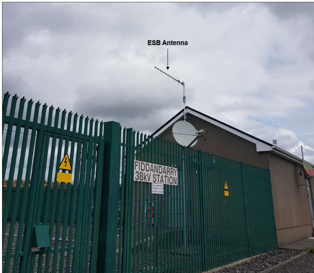
Figure 3. ESB Antenna at Fiddandarry Substation
